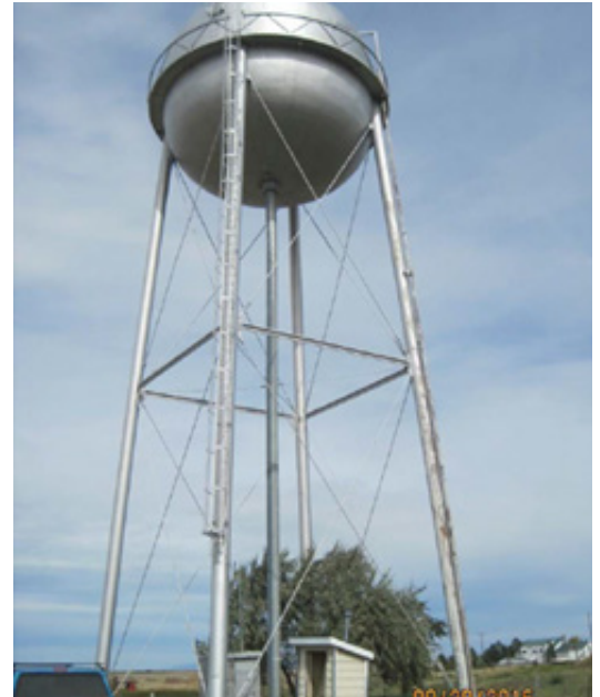
Figure 10 Elevated Steel Water Ta
