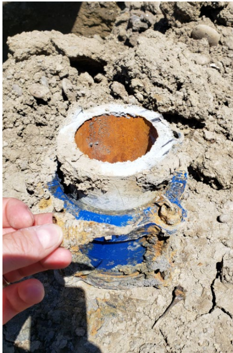
Figure 3 - Removed coupler to AC main (notice completed corroded bolt in the hand)
