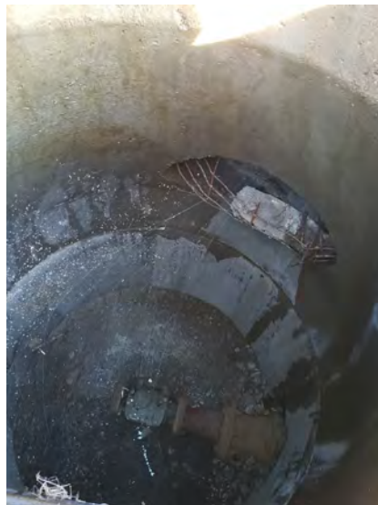
Figure 3-3 - Main Meter Vault
