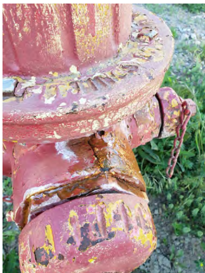
Figure 3-10 - Corroded and Leaking Hydrant in Geraldine
