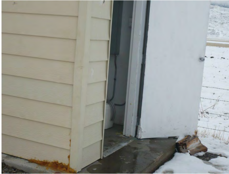
Figure 3-4 - Picture of Chlorine Treatment Building with Sealant Applied to Stop Rodents
