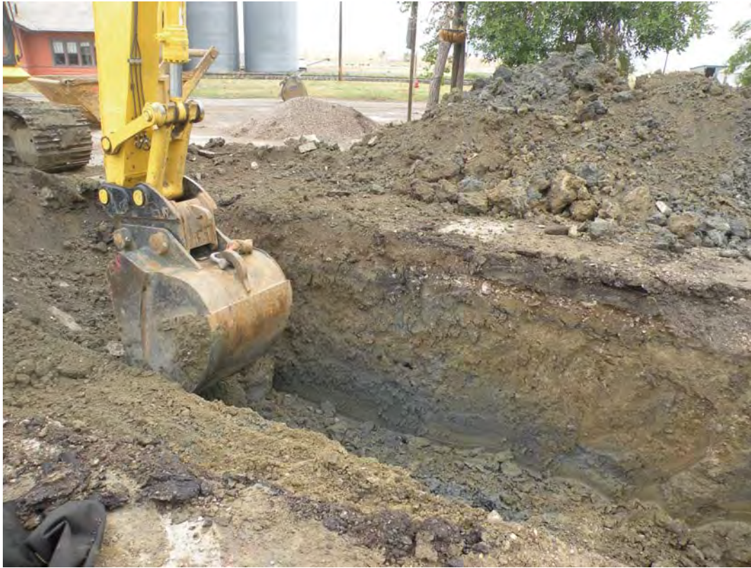
Stained soil, northern impacted area.
