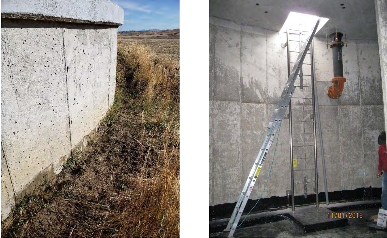
Figure 3-5 - Pictures of the Exterior (left) and Interior (right) of the Concrete Tank
