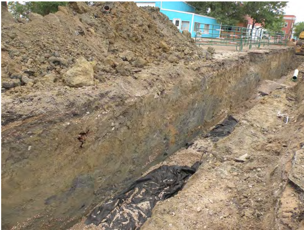
Northern impacted area looking south. Samples SW1 4-7 and SW1 7-8 collected at lower center of photo.
