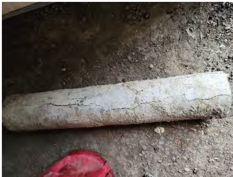
Figure 3-8 - Typical AC Water Main with Fractures
