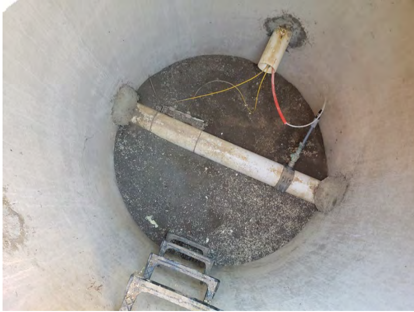
Figure 3-2 - Chlorine Injection Vault with the Flow Meter (Left) and the Injection Quill (Right)
