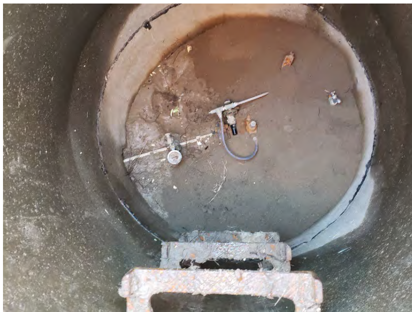
Figure 3-6 - Soil Intrusion into PRV Vault
