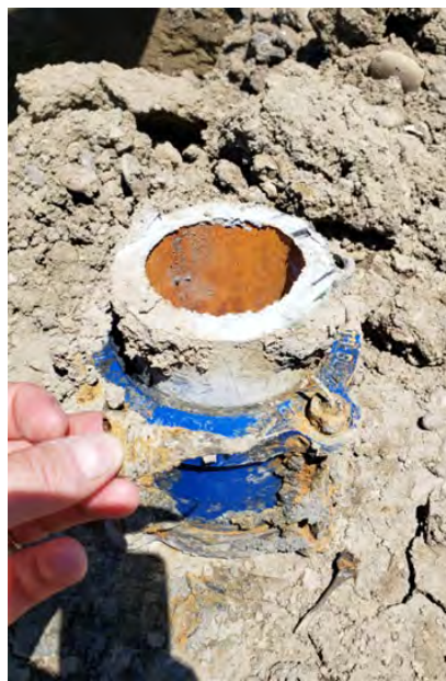
Figure 3-9 - Corroded Water Coupler to AC Main
